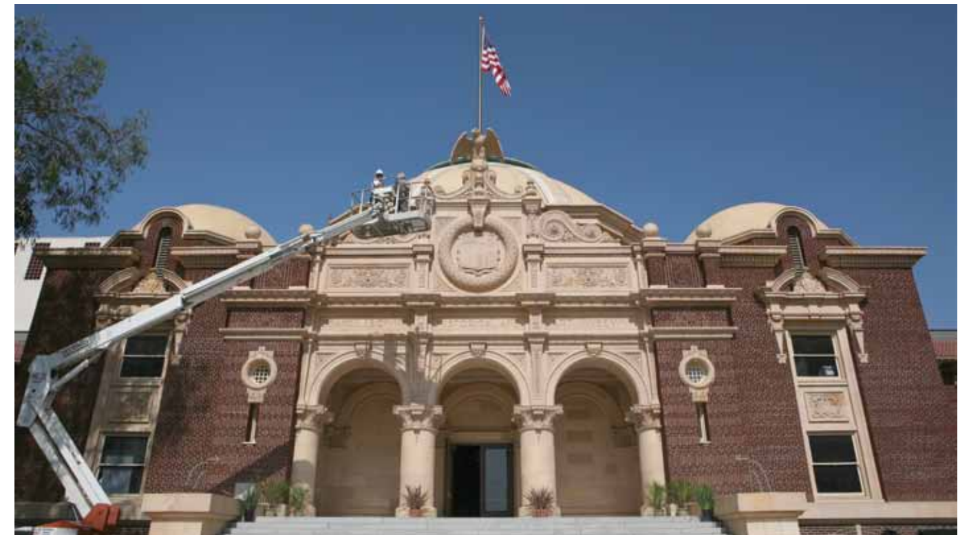
L.A. County Second District Supervisor Mark Ridley-Thomas heads upward to partake in the unveiling of the 1913 Building's recreated eagle.
